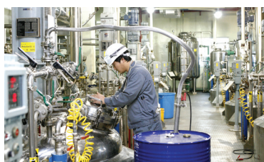
ST Pharm Plant
